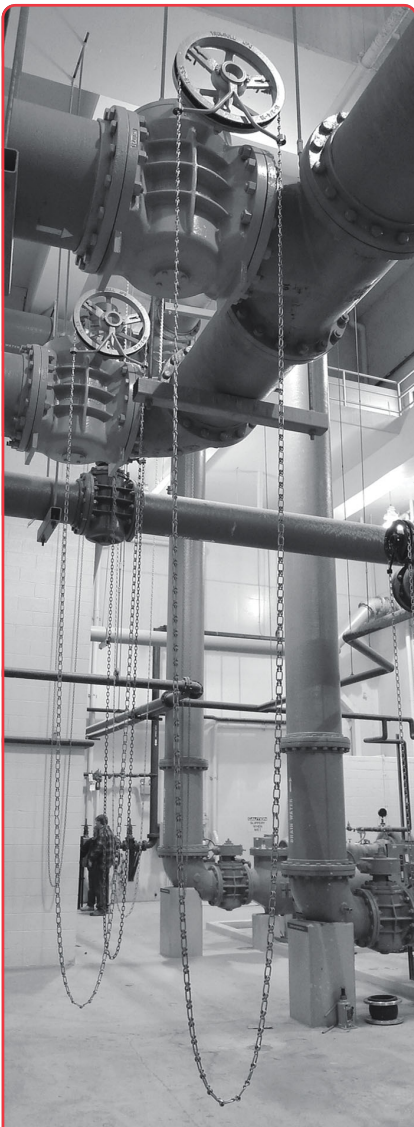
CHAIN FROM OVERHEAD CHAINWHEEL SHOWN IN PATHWAY.
